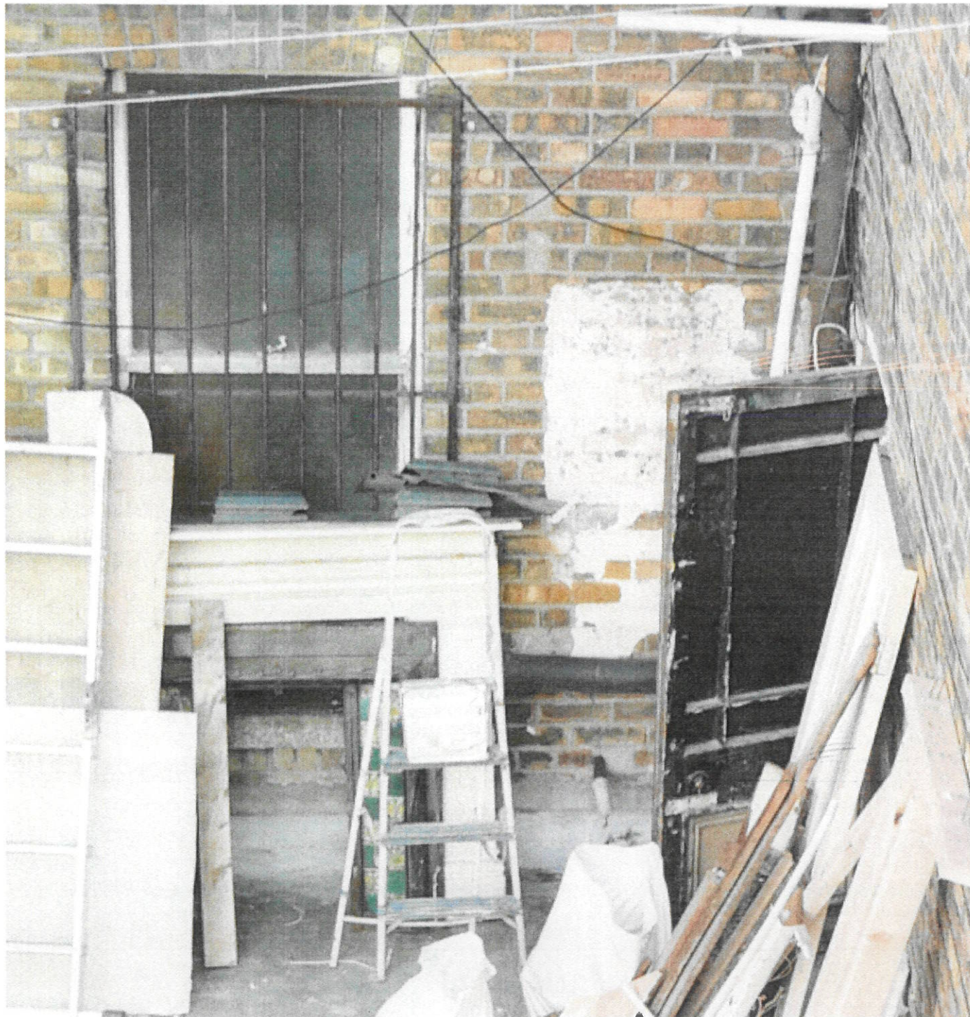
B = Dining room window & C = Timber door to the “roof area for guest’s”
