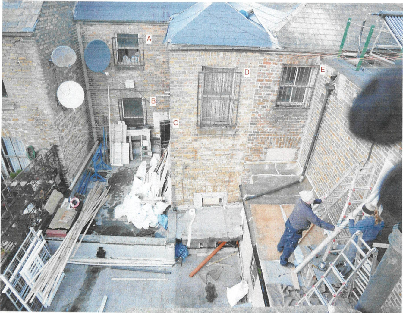
6.3 Rear view of the Lamplighter Public House on the day of the dismantling of my spiral staircase in January 2018:
